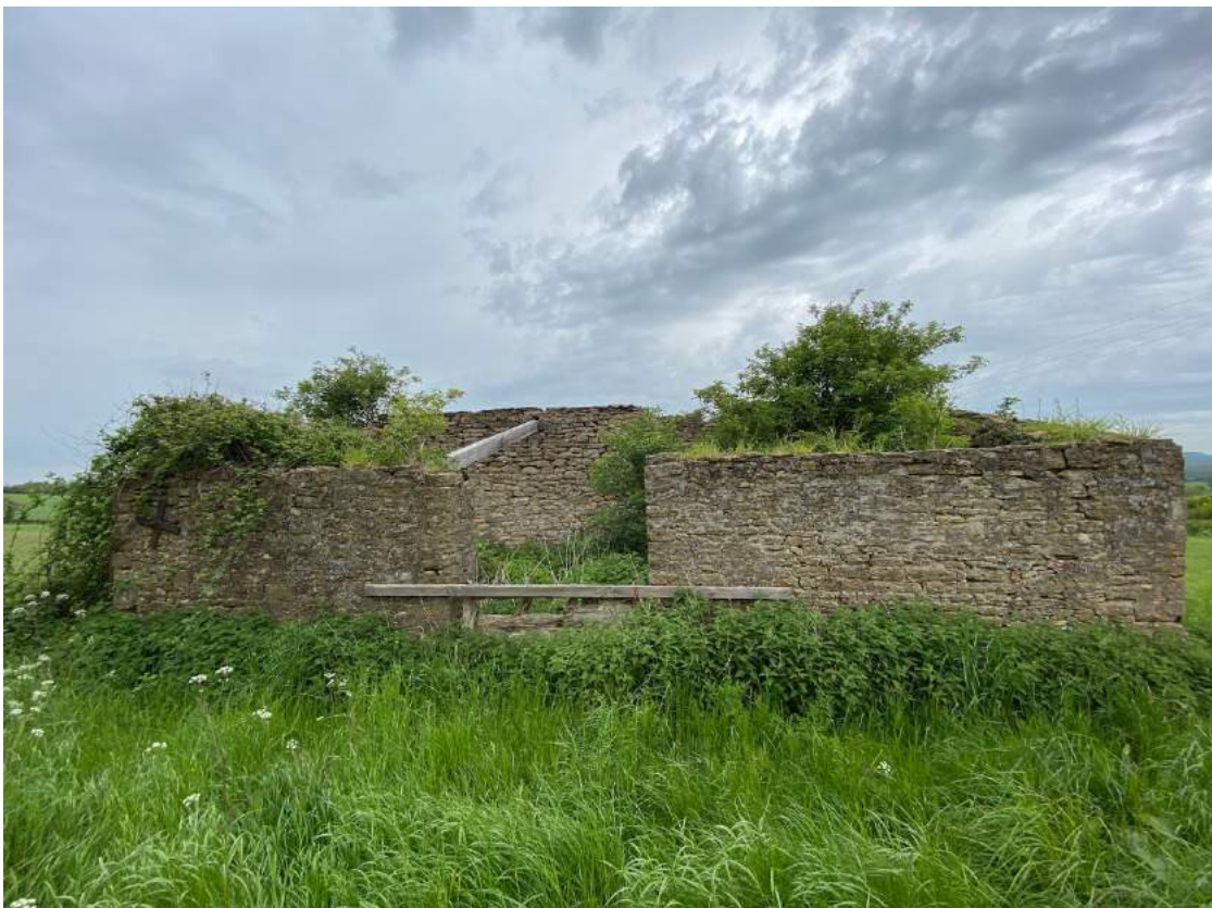
Dilapidated building within F7
